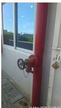
Fire System Valve.jpeg
